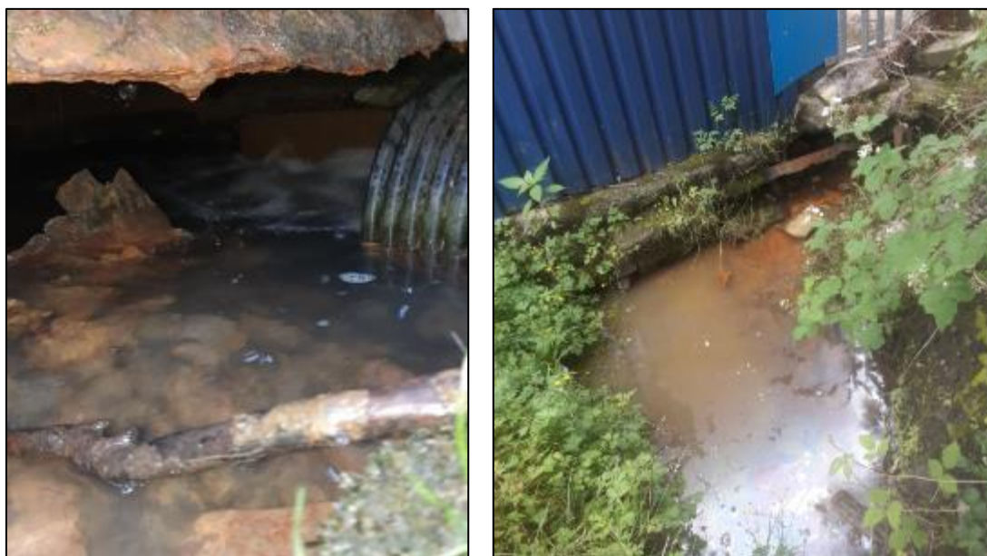
Figure 13: Outfall pipe entering 'Culvert Inlet 2' (left) and standing water surrounding 'Culvert Inlet 2' (right) (captured during CCTV survey operations on 30/06/2020)
