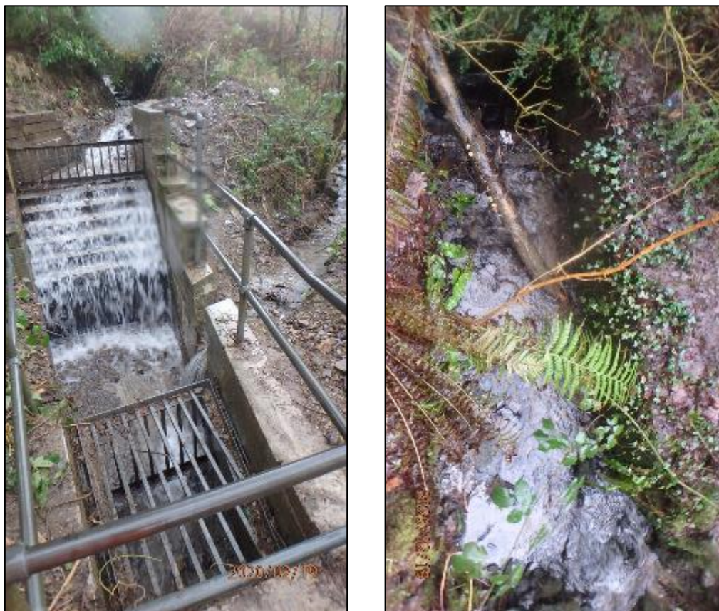
Figure 10: 'Culvert Inlet 5' (left) and 'Culvert Inlet 6' (right) located to the rear of Tyn-y-coedcae which surcharged during Storm Dennis (captured by RCT's Flood Risk Management team on 19 th February 2020)
