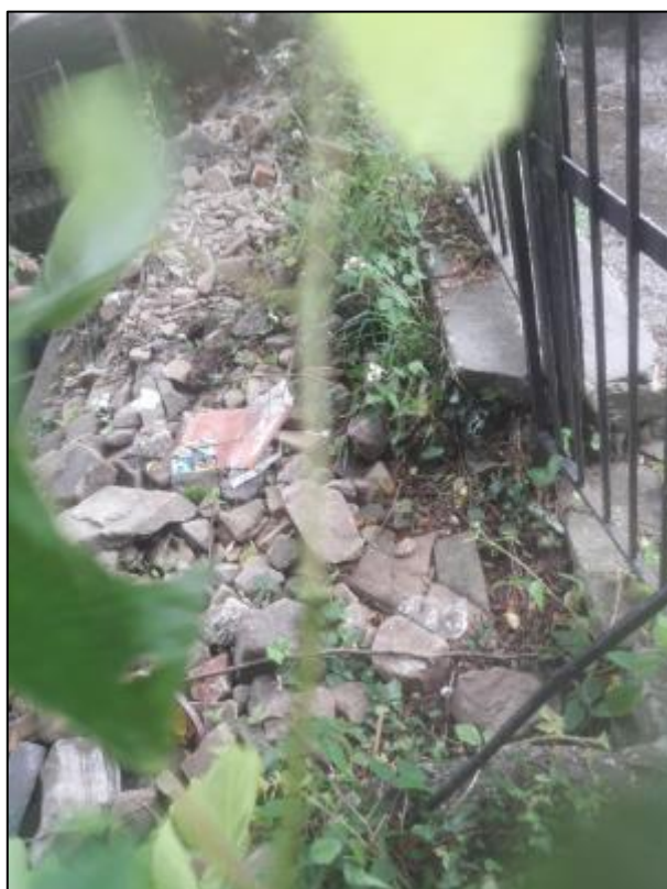
Figure 16: Debris removed from the 'Dumfries Street Culvert Network' during cleansing operations (image captured on 29/06/2020)
