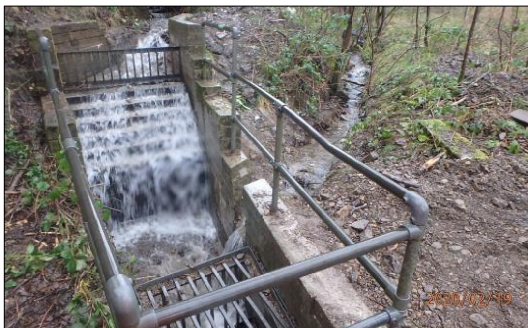
Figure 18: Photo of 'Culvert Inlet 6' captured by RCT's Flood Risk Management team following debris clearance post Storm Dennis (19/02/2020)
